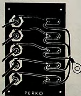
BACK VIEW OF IMPROVED PANEL
